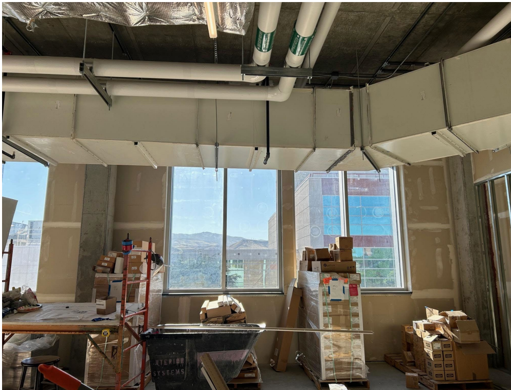
Fig. 3: Unfinished Space and Exposed Utilities of Third Floor to Be Completed in FY2026
