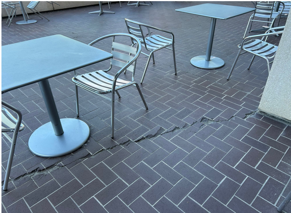
Fig. 2: Exterior Structural Damage
